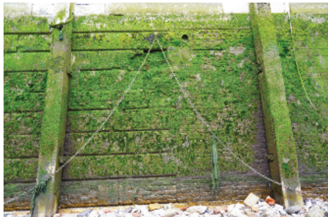
Examining the exterior wall area for The Arches reveals the state of disrepair.
