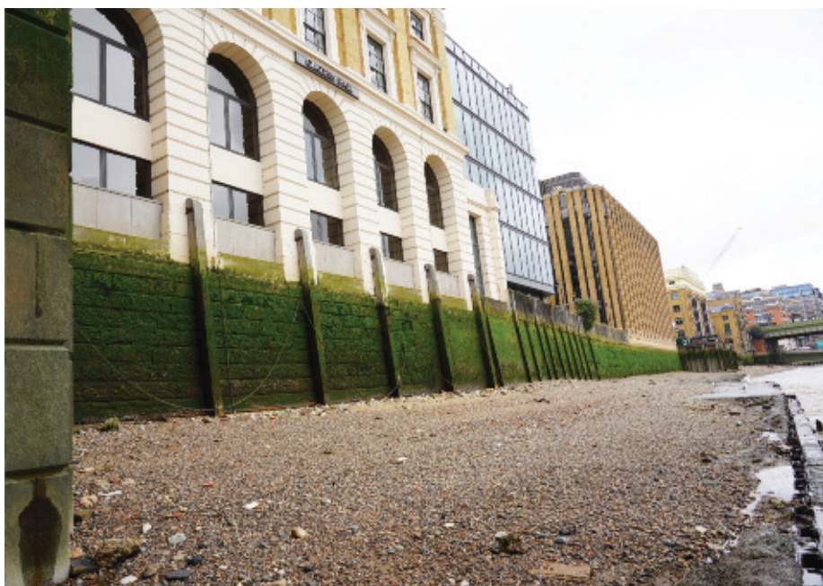
With the tide out the scale of Glaziers Hall's wall situation is revealed in full.
