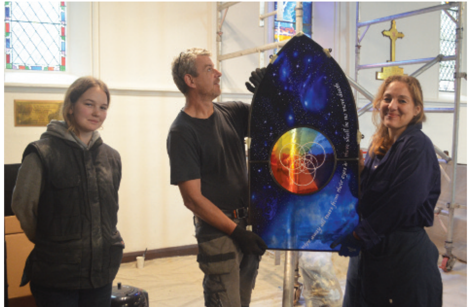
Installation of the window at All Saints Church, Dunsden Green required collaboration – so here are Dan Humphries and his colleague India Savill with Natasha (right).
